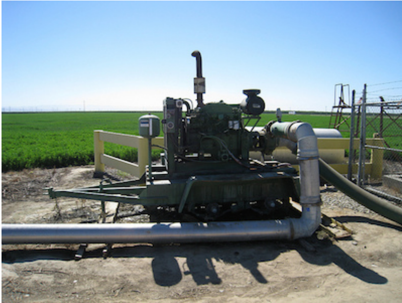
Groundwater irrigation in California's Central Valley. Photo used with permission from Chris Austin of mavensnotebook.com .
