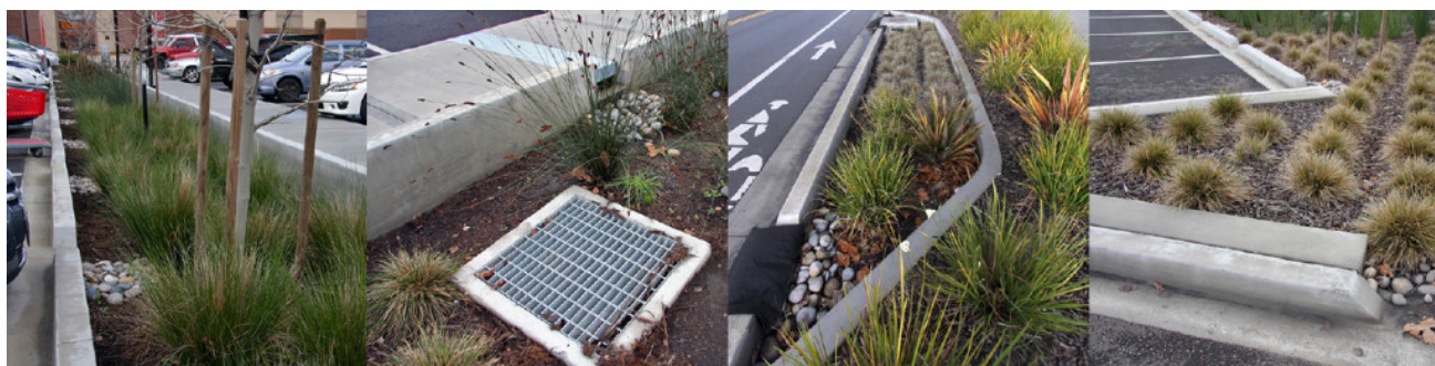
Green stormwater infrastructure includes bioretention systems. (Photos by Nell Green Nylén)
