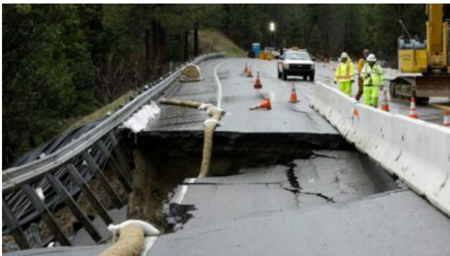
The westbound lane of Highway 50 (near Pollock Pines, towards Lake Tahoe) collapsed in February 2017.
