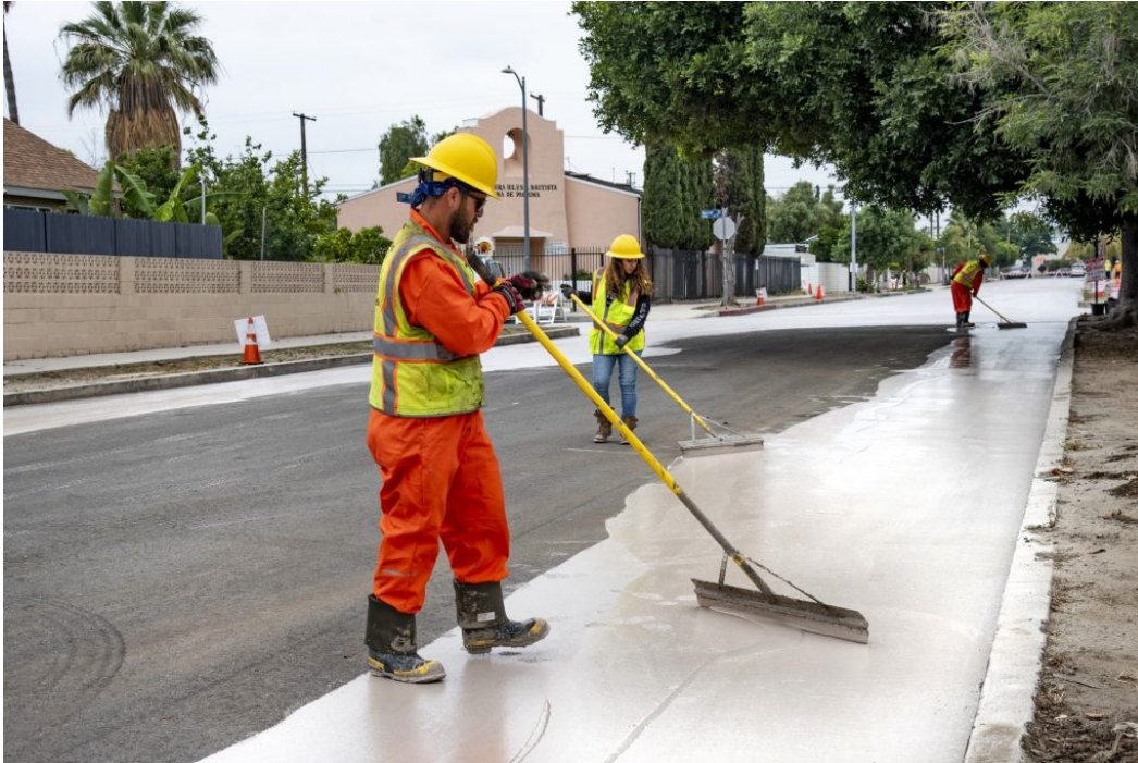
Los Angeles city workers install a cool pavement treatment in Pacoima. Photo credit: City of Los Angeles Bureau of Street Services
