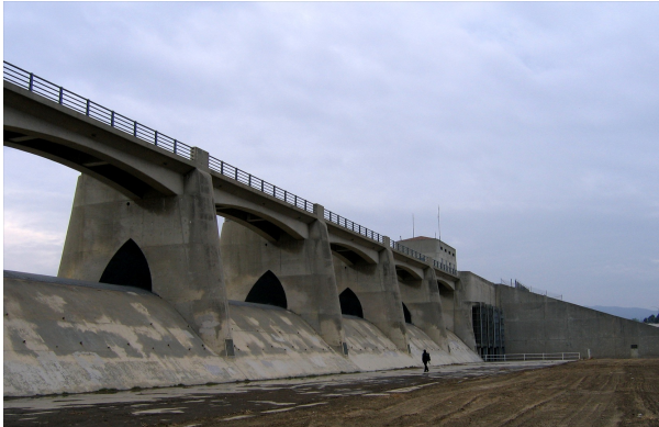
Sepulveda Dam, which withholds winter flood waters along the Los Angeles River. Courtesy Flickr .
